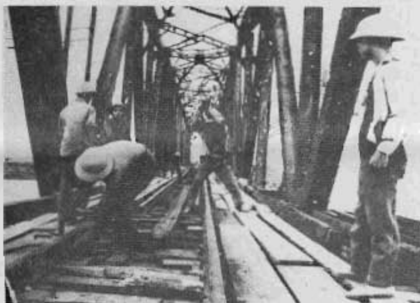
Work brigades rebuild a bridge along Highway One destroyed by Saigon bombing
